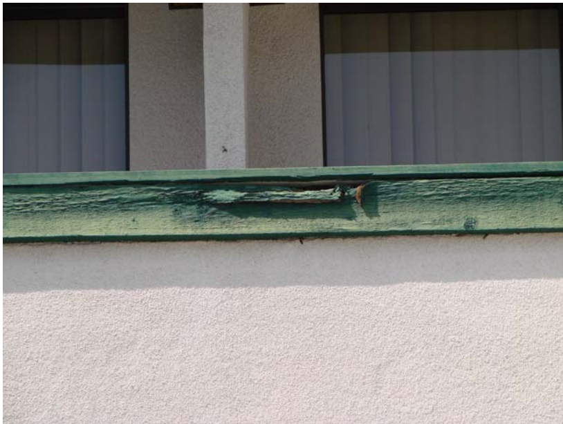
184 P_E: Detail - rotten wood trim on 2nd floor balconies.
