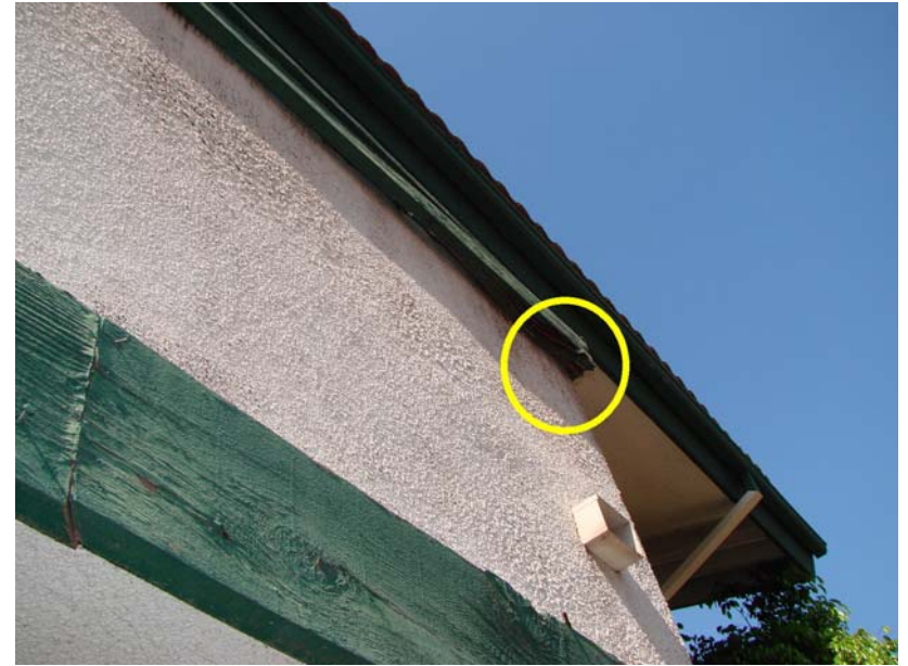
071 P_W: Detail - rotten wood trim on 2nd floor balconies.
