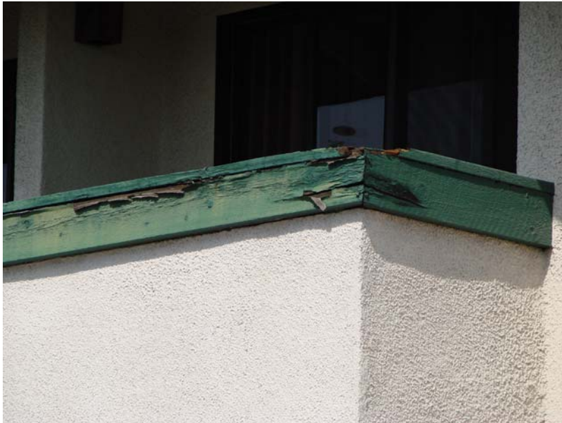
034 P_E: Detail - rotten wood trim on 2nd floor balconies.
