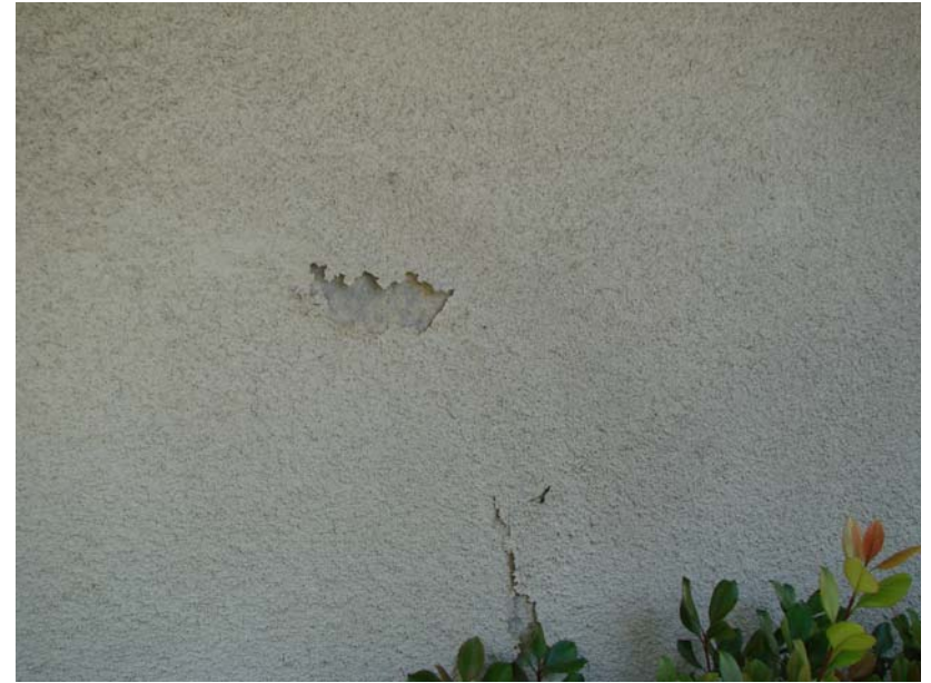
067 P_W: Exterior finish coming off building.
