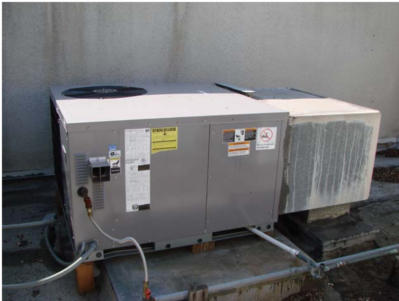
060 P_W: Heil HVAC unit in roof well - AC & gas heat.
