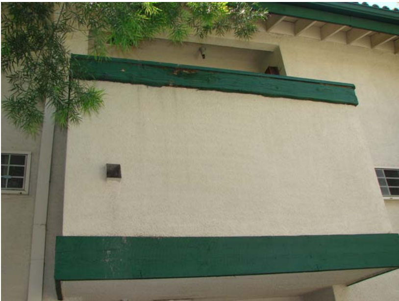
176 P_E: Detail - rotten wood trim on 2nd floor balconies.
