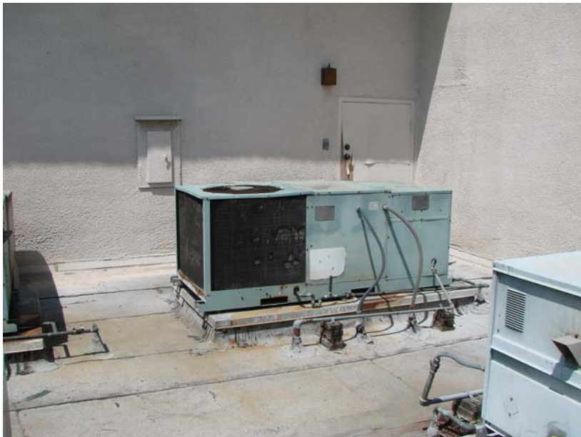
152 P_E: Rooftop HVAC unit - AC & gas heat.
