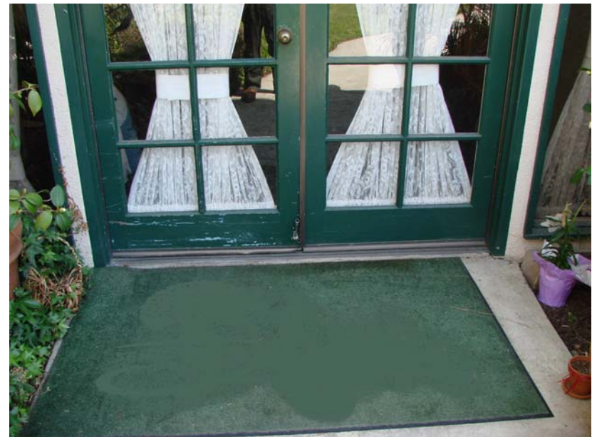
157 P_E: Detail - courtyard doors need repainting.
