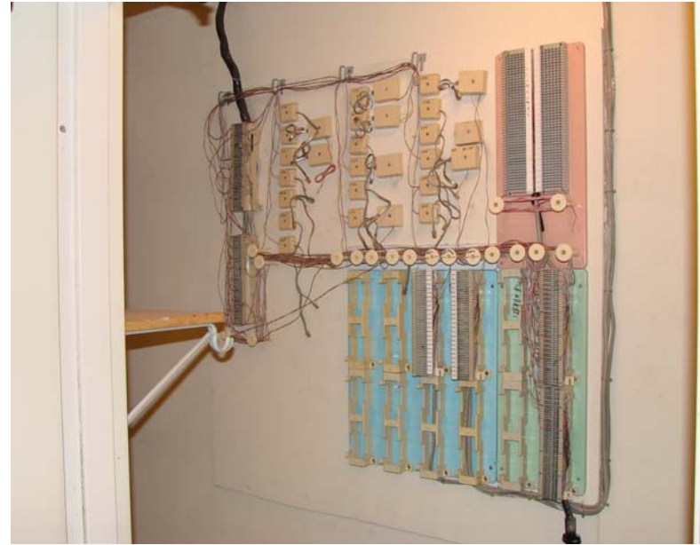
139 P_E: 2nd floor electric closet - telephone patch panel.
