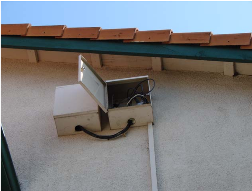
048 P_E: Open CATV junction box.
