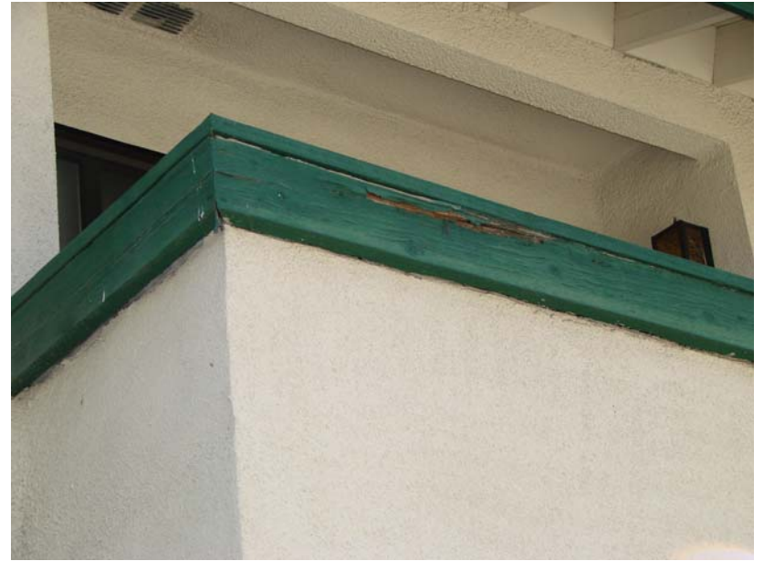
183 P_E: Detail - rotten wood trim on 2nd floor balconies.
