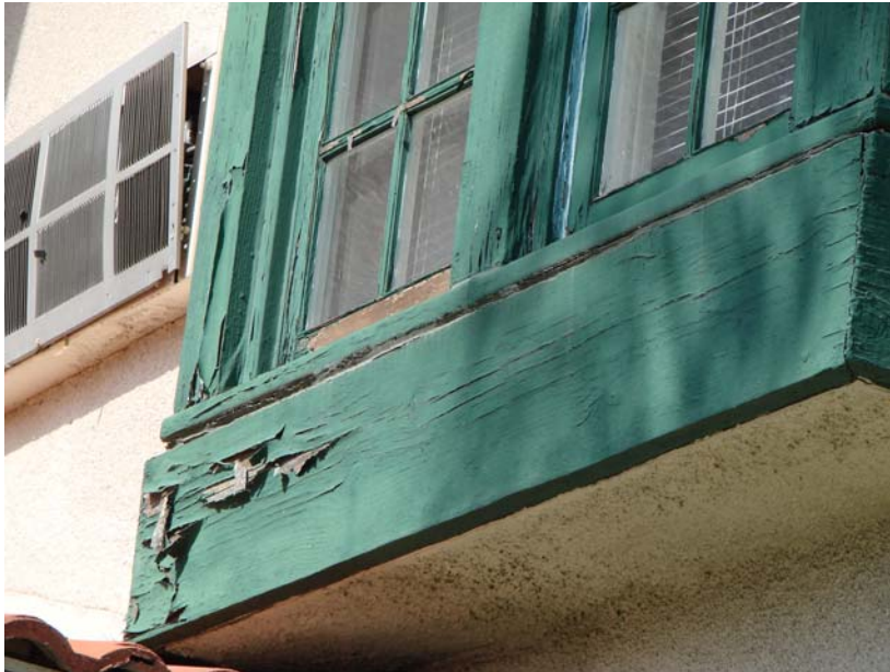
090 P_W: Rotten wood trim on windows.
