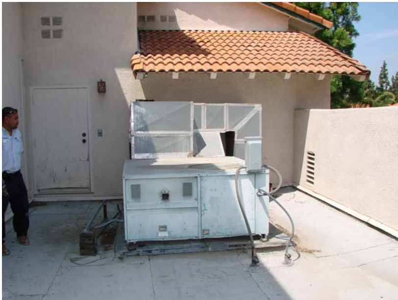
140 P_E: Palm East - Carrier Weathermaker rooftop HVAC unit - AC & gas heat.
