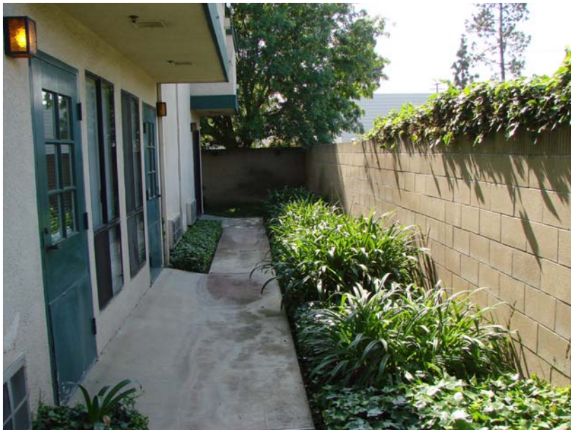
076 P_W: Sidewalk detail - slopes away from building, appears to pond some water.
