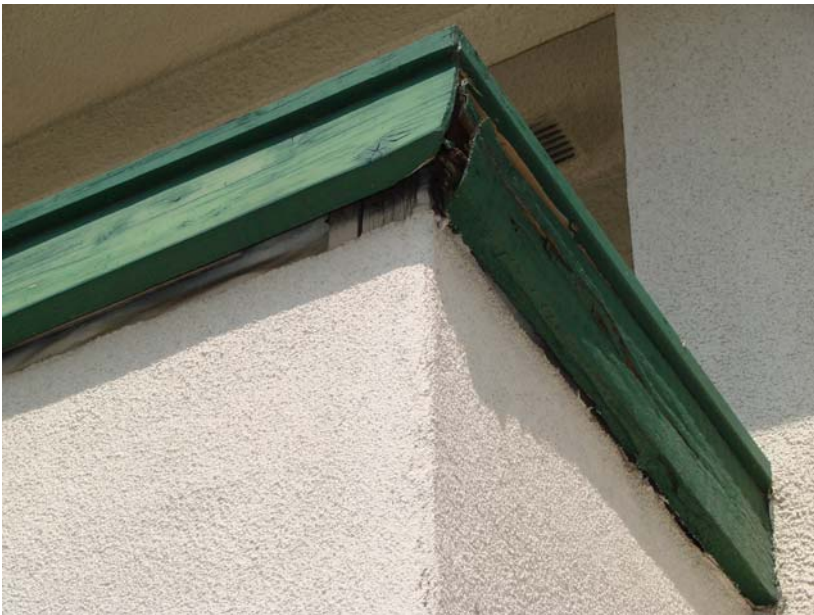
188 P_E: Detail - rotten wood trim on 2nd floor balconies.
