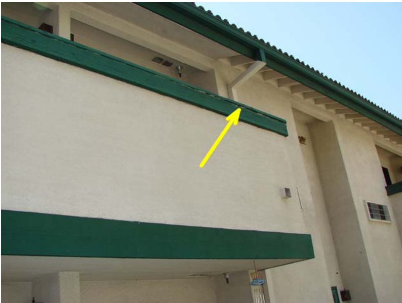
180 P_E: Detail - rotten wood trim on 2nd floor balconies.
