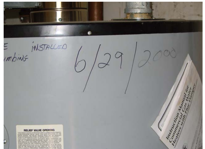
093 P_W: State water heater (#2), 100-gal, 260,000 BTUH.
