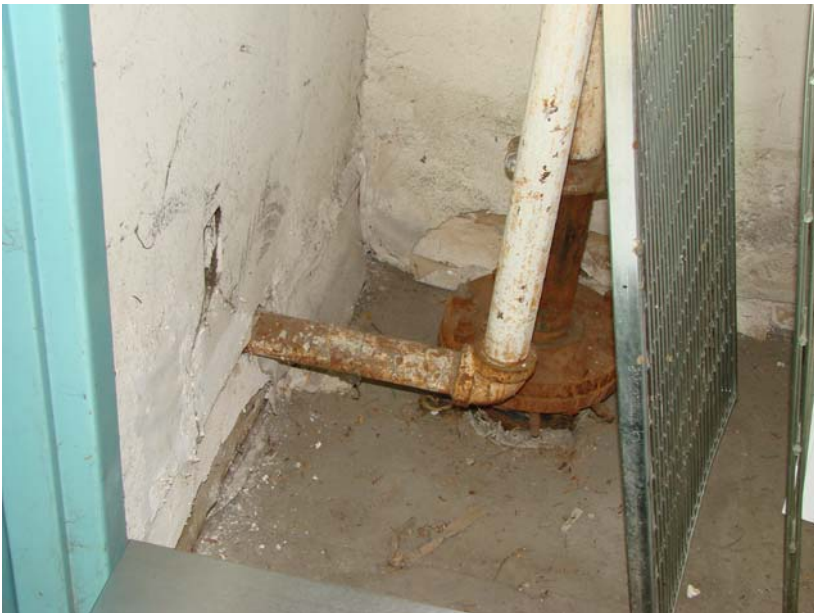
032 P_E: Water damage in water heater closet.
