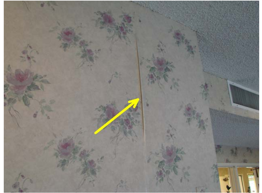
031 P_W: Living room - peeling wallpaper.
