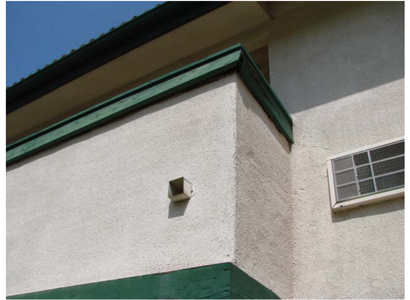
187 P_E: Detail - rotten wood trim on 2nd floor balconies.
