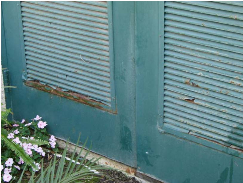
168 P_E: Detail of elevator equipment room doors - doors will need to be replaced in future years.
