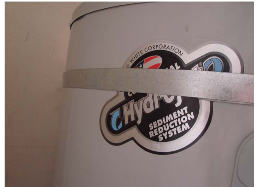
025 P_E: Bradford White water heater (#1) 100-gal, 270,000 BTUH.
