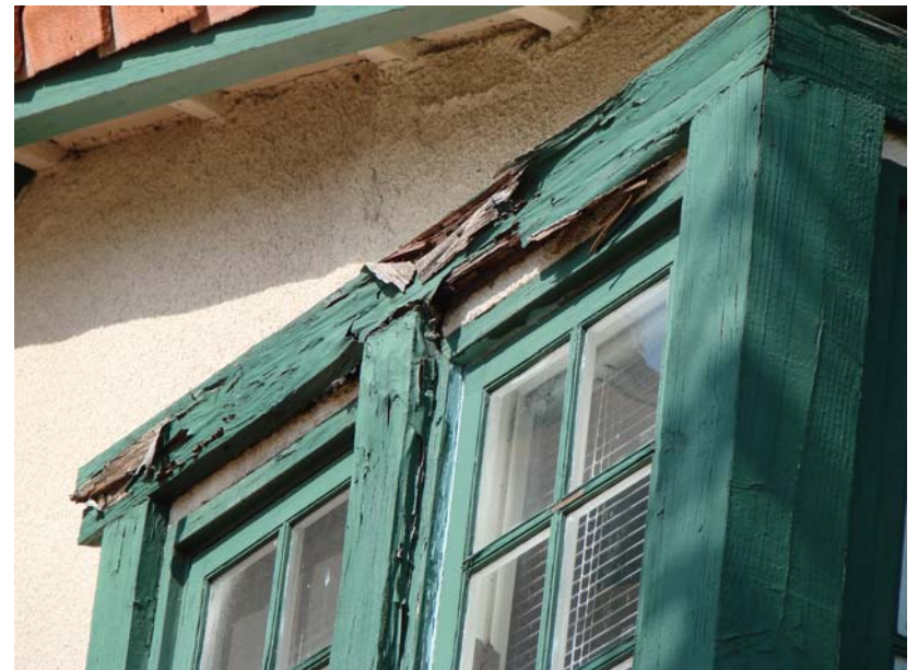
089 P_W: Rotten wood trim on windows.
