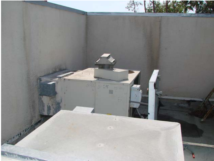
058 P_W: Day & Night HVAC unit in roof well - AC & gas heat.
