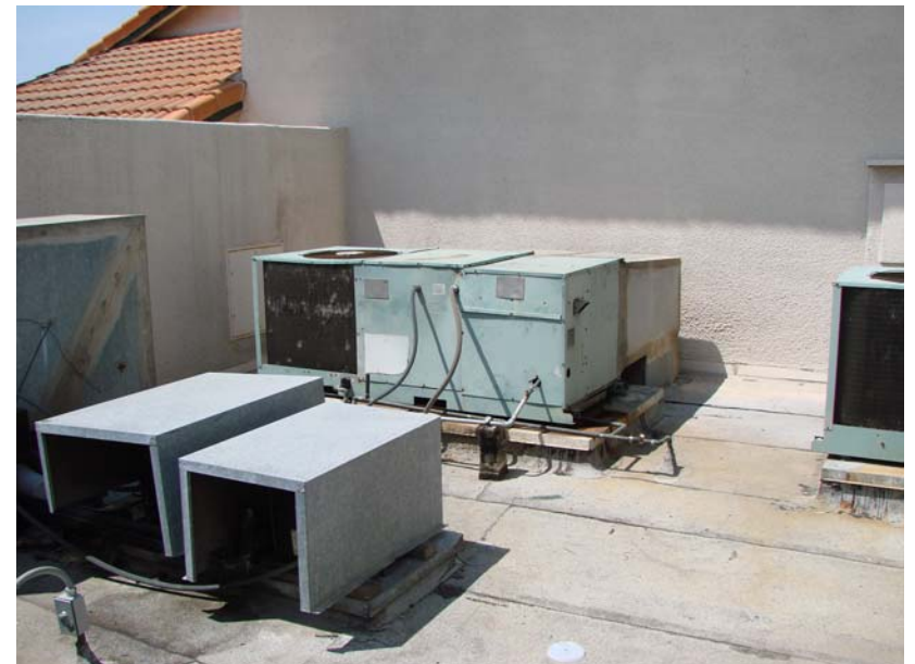
149 P_E: Rooftop HVAC unit - AC & gas heat; Kitchen walk-in cooler-freezer compressors.
