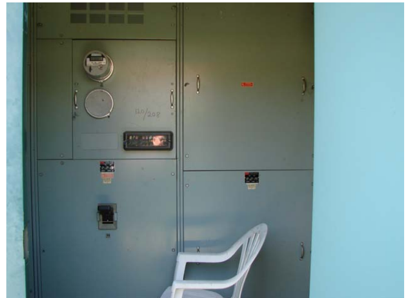
037 P_E: 2000 Amp main electric panel (Palm East).
