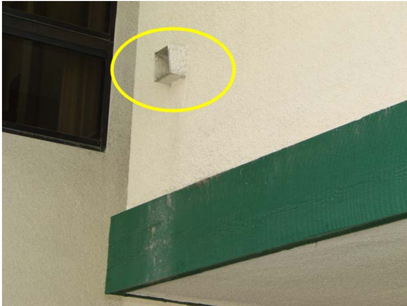
178 P_E: Detail - balcony drain. Consider adding drain scuppers to extend runoff beyond balcony wall.
