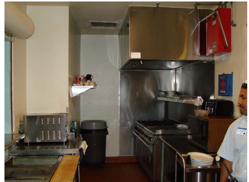
017 P_W: Kitchen - Wolf 6-burner stove with griddle and double oven.
