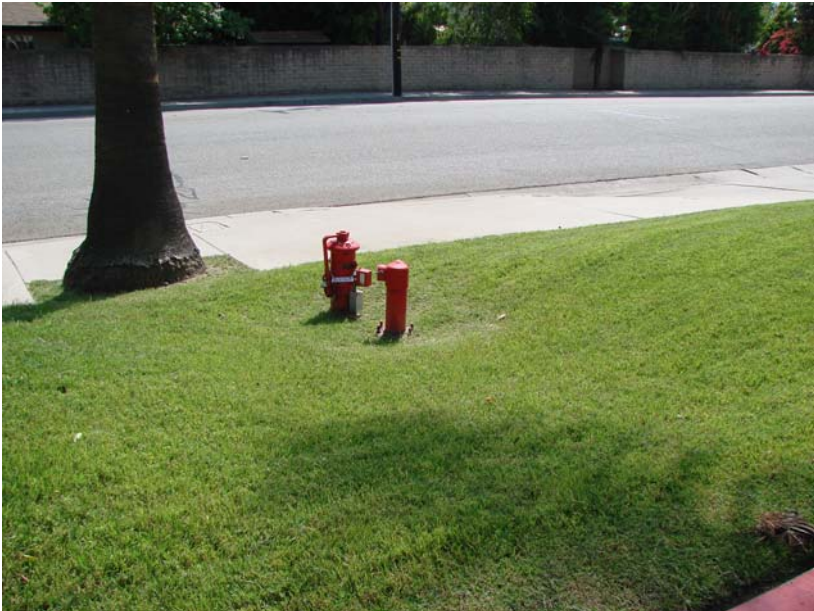
012 P_E: Fire sprinkler stand pipe.
