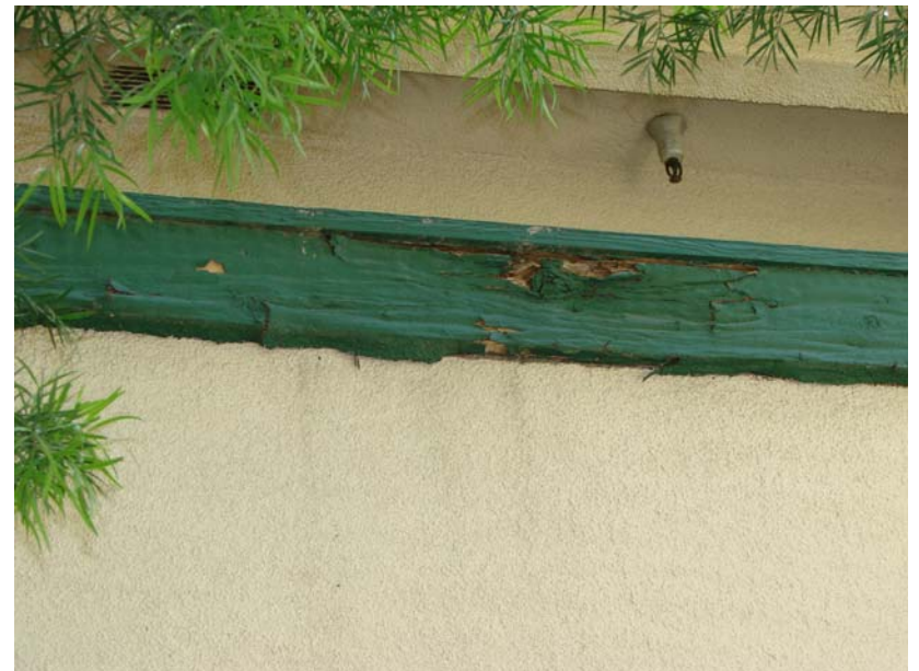
177 P_E: Detail - rotten wood trim on 2nd floor balconies.
