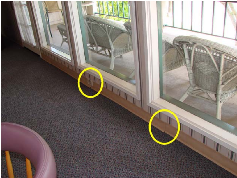
048 P_W: Detail - poor floor base installation.
