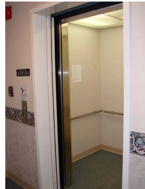
041 P_W: Elevator interior detail.
