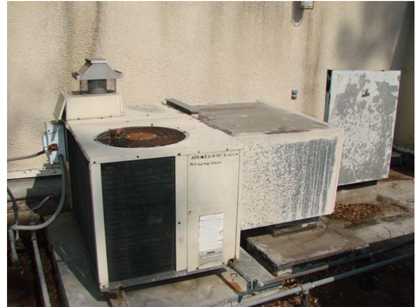
063 P_W: Day & Night HVAC unit in roof well - AC & gas heat.
