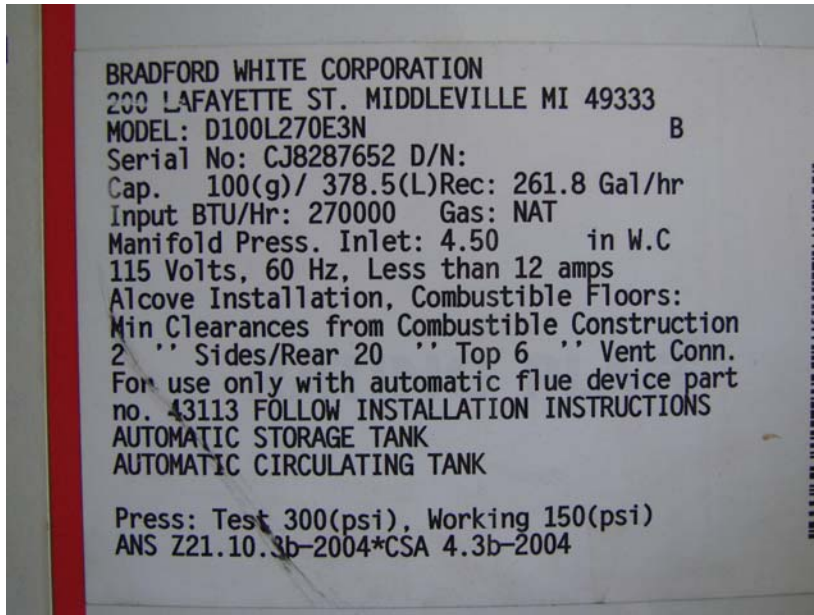
026 P_E: Bradford White water heater (#1) 100-gal, 270,000 BTUH.
