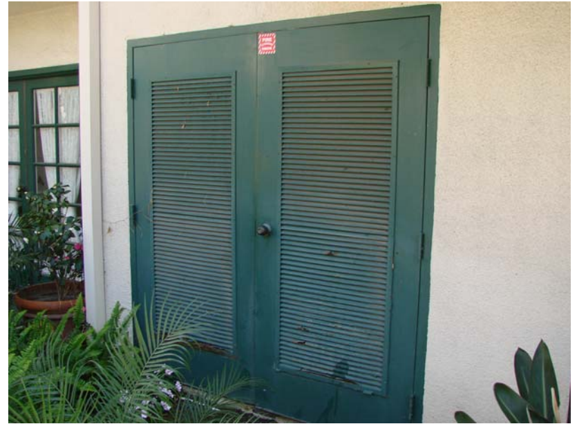
167 P_E: Elevator equipment room in courtyard.
