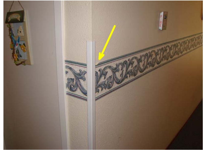
087 P_E: Detail - wallpaper border peeling at wall corner. (Note - staff has not yet begun 1st floor painting improvements.
