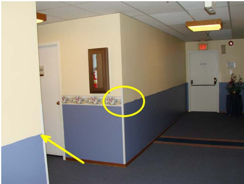
124 P_E: 2nd floor east hall @ north end. Note missing wallpaper border - staff in the process of installing border after painting corridor walls.
