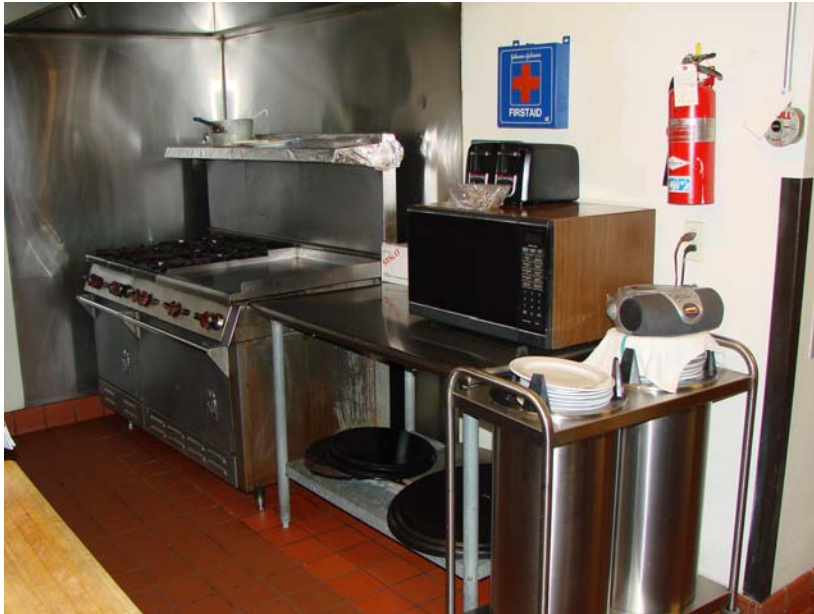
018 P_W: Kitchen - Wolf 6-burner stove with griddle and double oven.
