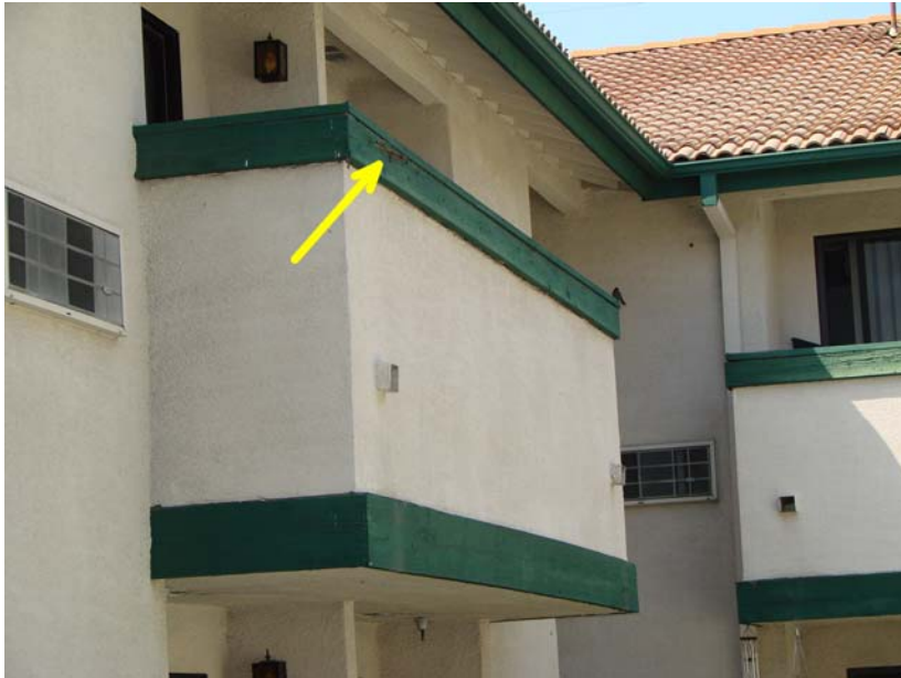
182 P_E: Detail - rotten wood trim on 2nd floor balconies.
