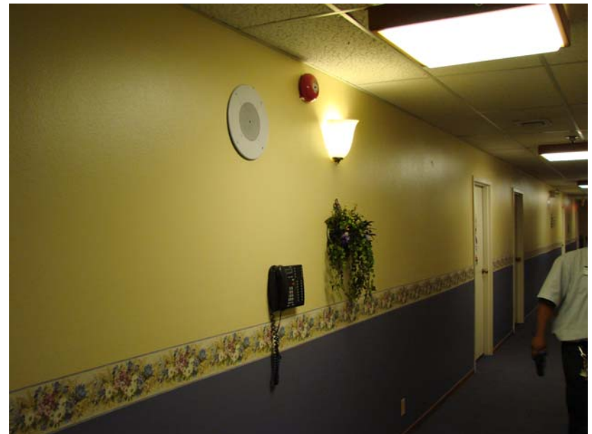
117 P_E: Public Address speaker, fire alarm, house phone - 2nd floor West Hall.
