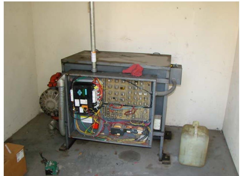
169 P_E: Hydraulic elevator equipment - recent repairs-maintenance.
