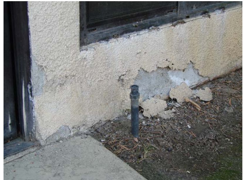
171 P_E: Water damage detail.
