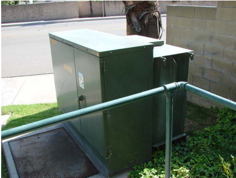
086 P_W: Pad mounted electrical transformer.
