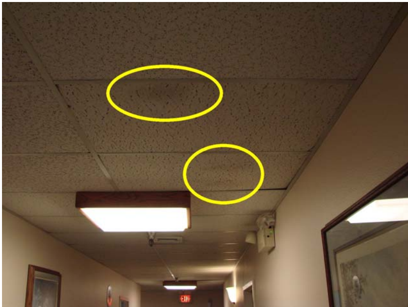
088 P_E: Darks spots on ceiling tile - consider repainting grid and replacing-painting ceiling tile.
