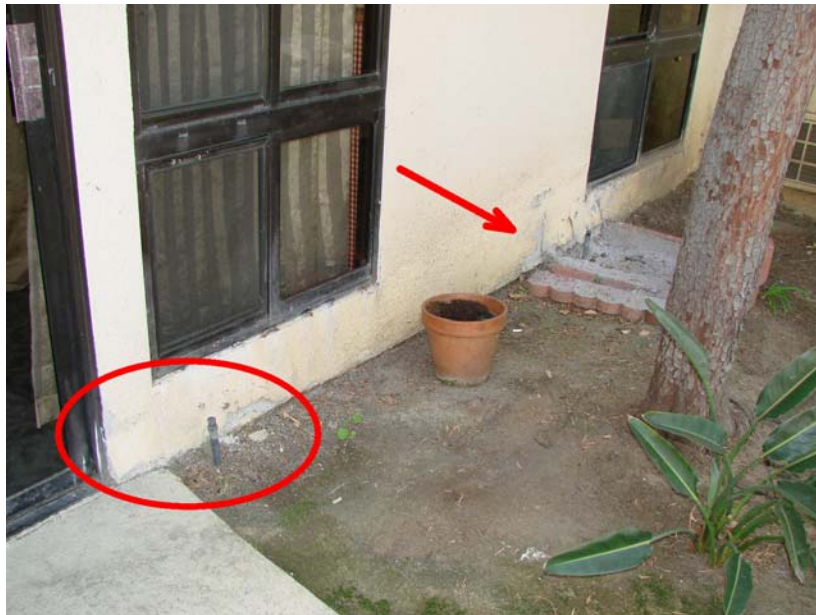
170 P_E: Courtyard detail - water damage outside private dining room (possibly from sprinklers-).
