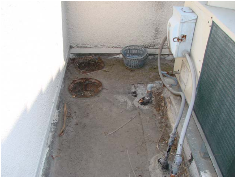
056 P_W: Roof drain in roof well - note drain covers out of place.
