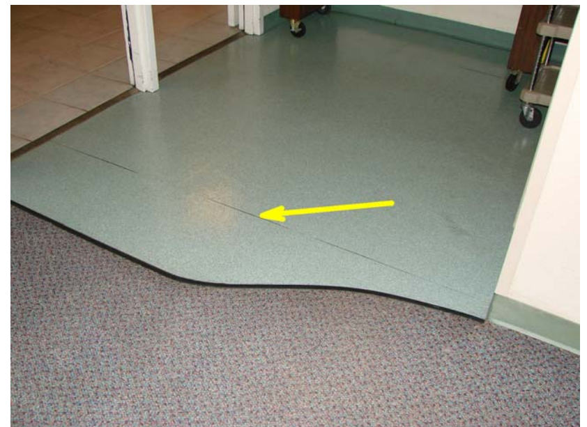
013 P_W: Dining room floor detail - note separated seam in sheet vinyl.
