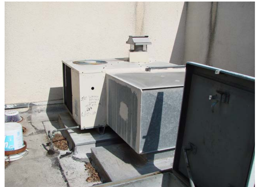
057 P_W: Day & Night HVAC unit in roof well - AC & gas heat.
