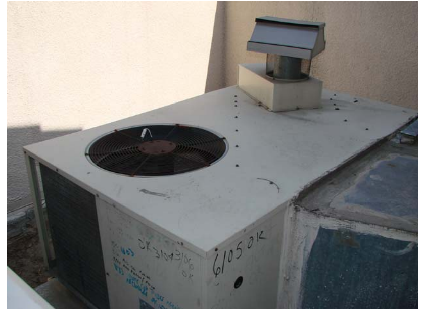
055 P_W: Payne HVAC unit (AC & gas heat) in roof well.
