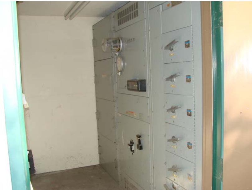
084 P_W: Main electric service - 1000 Amp main panel.
