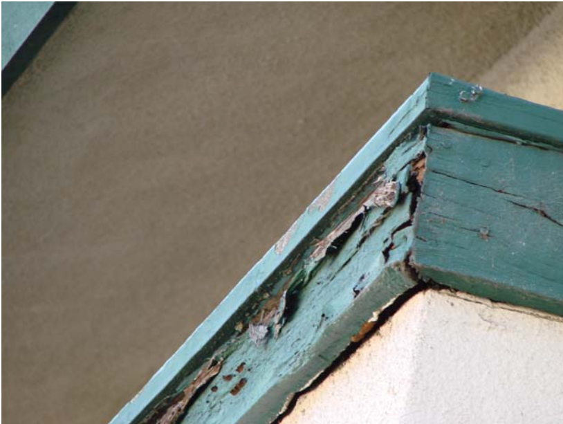
044 P_E: Detail - rotten trim on 2nd floor balcony.
