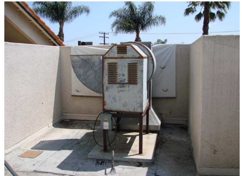
145 P_E: Kitchen air handler.
