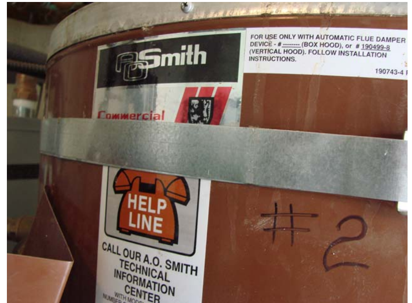
023 P_E: A.O. Smith water heater (#2) - 100-gal, 250,000 BTUH.
