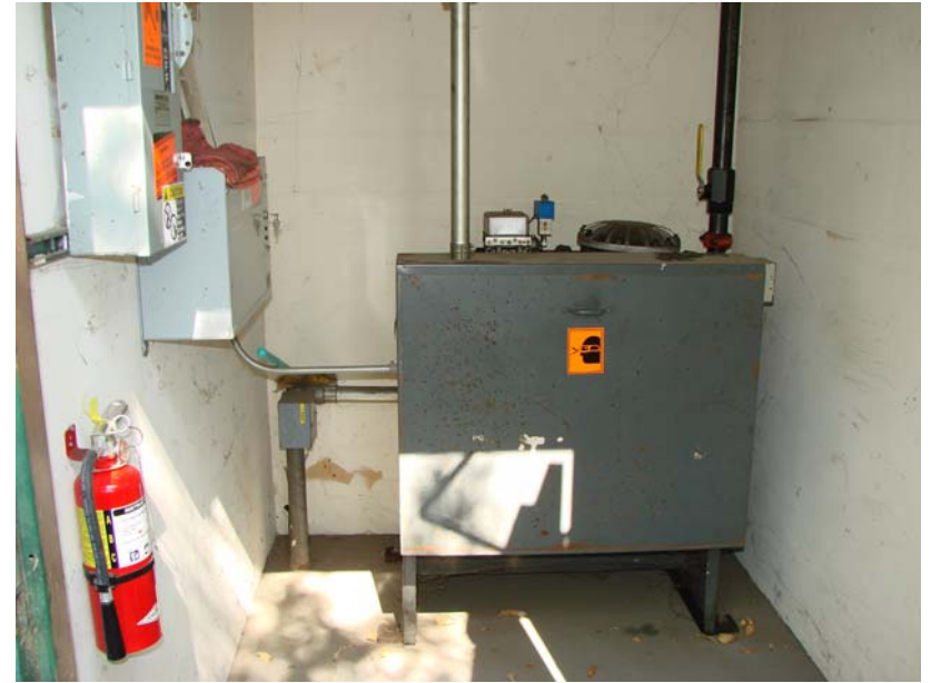
083 P_W: Hydraulic elevator equipment room.
