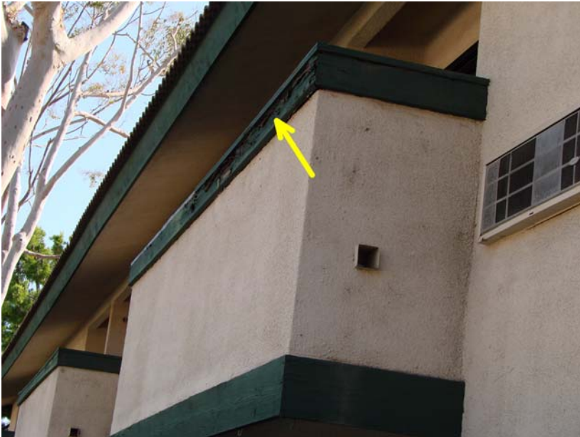
042 P_E: Detail - rotten trim on 2nd floor balcony.
