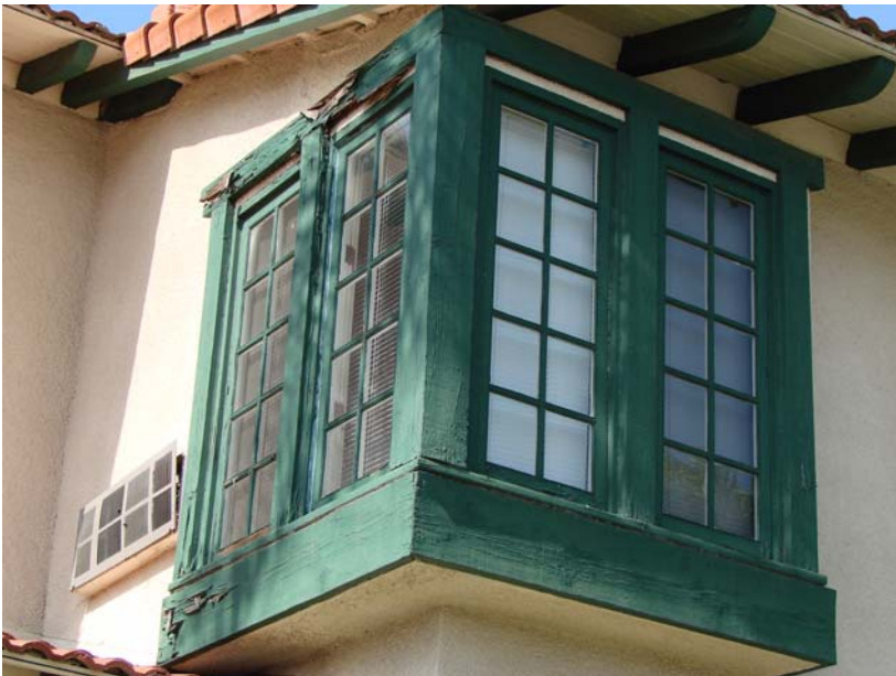
088 P_W: Rotten wood trim on windows.
