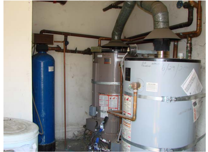
091 P_W: American Standard & State 100-gallon water heaters with water treatment system.
