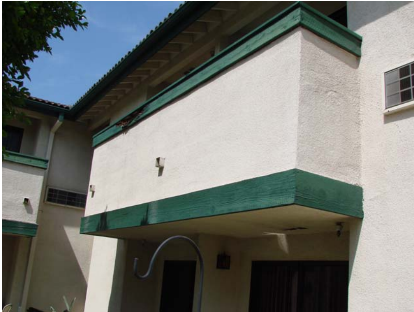
186 P_E: Detail - rotten wood trim on 2nd floor balconies.
