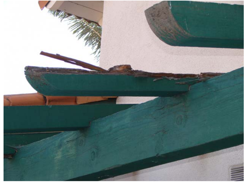
039 P_E: Detail - rotten beam.
