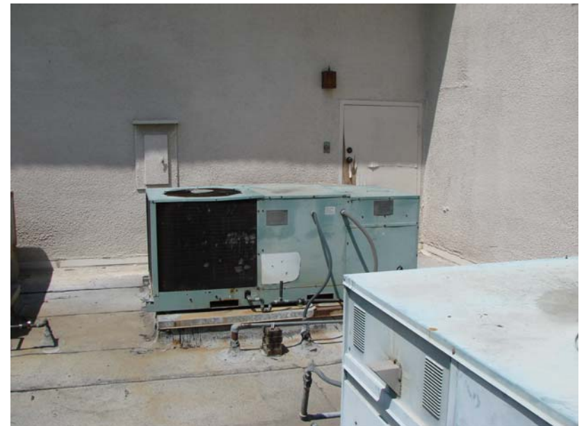
153 P_E: Rooftop HVAC unit - AC & gas heat.
