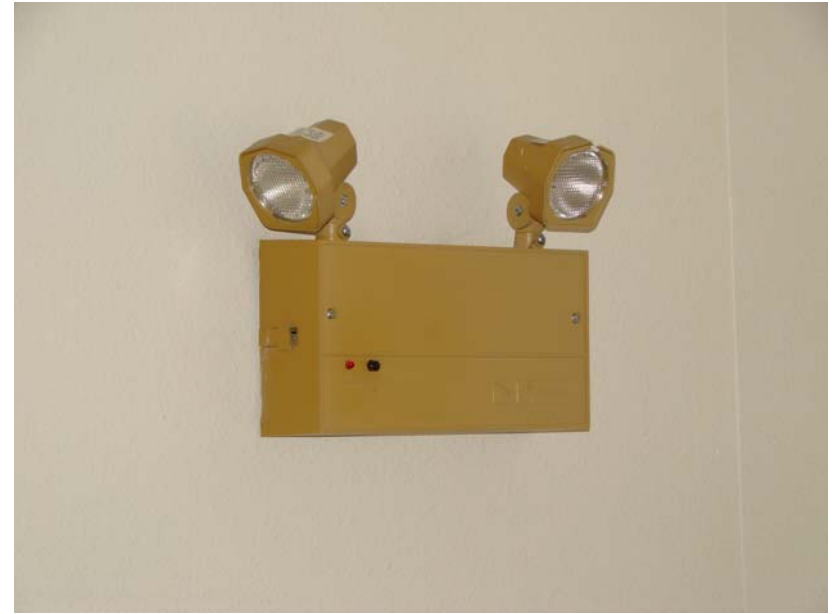
035 P_W: Original fixture - battery backup emergency lighting, some are being replaced.
