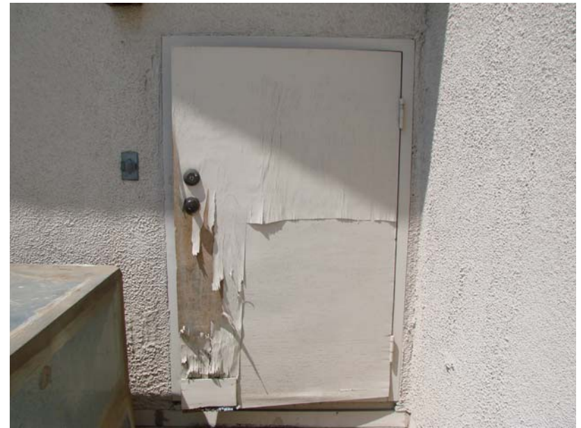
143 P_E: Roof well access door needs to be replaced.
