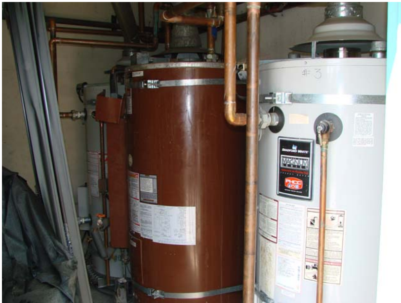
020 P_E: Water heaters - two for residential-domestic use; one for kitchen.
