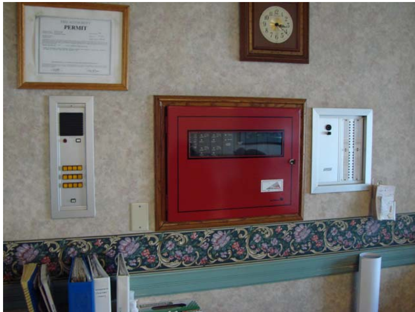
010 P_W: Palm West - Silent Knight fire alarm annunciator panel and Mirtone emergency-nurse call panel.
