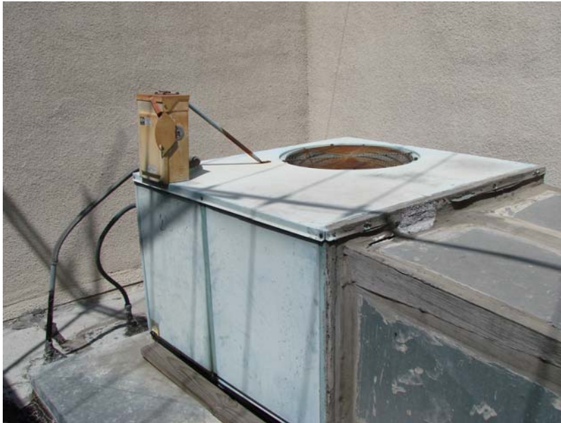
122 P_E: HVAC (AC & gas heat) unit in roof well above storage closet.
