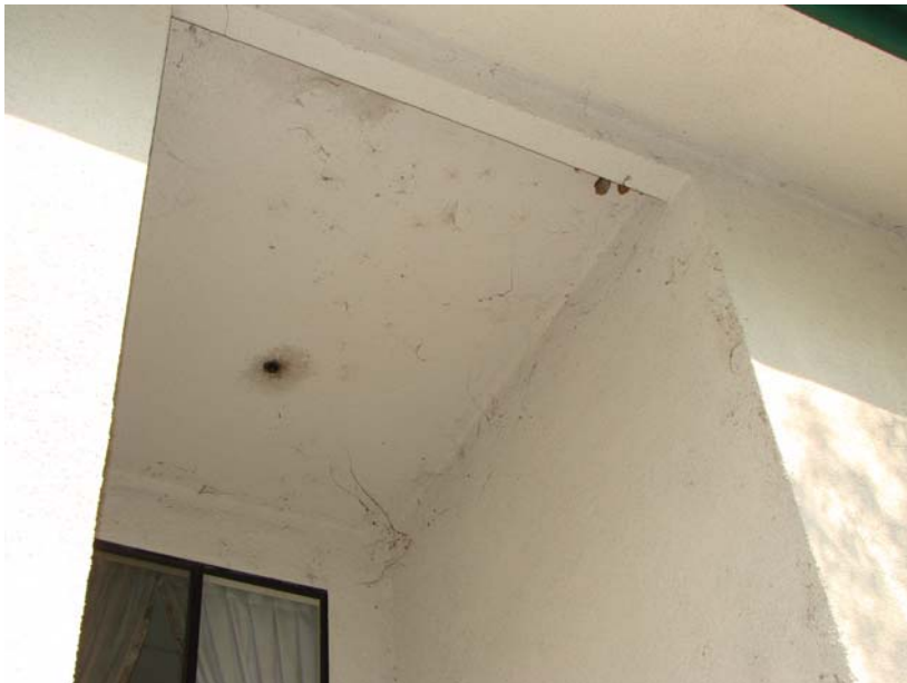
080 P_W: Spider webs in exterior alcove - building exterior should be pressure washed.
