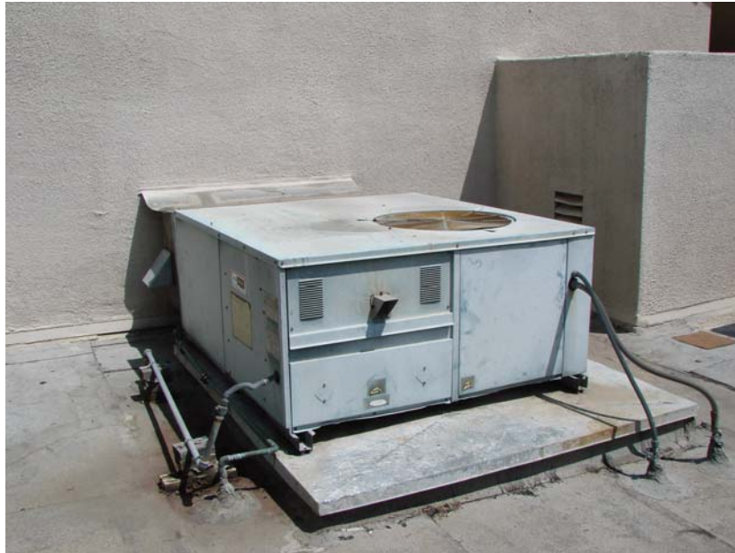
146 P_E: Carrier Weathermaker Rooftop HVAC unit - AC & gas heat.
