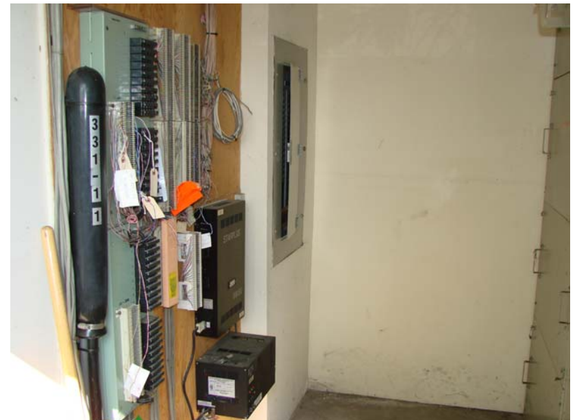
085 P_W: Main telephone patch panel in electrical room.
