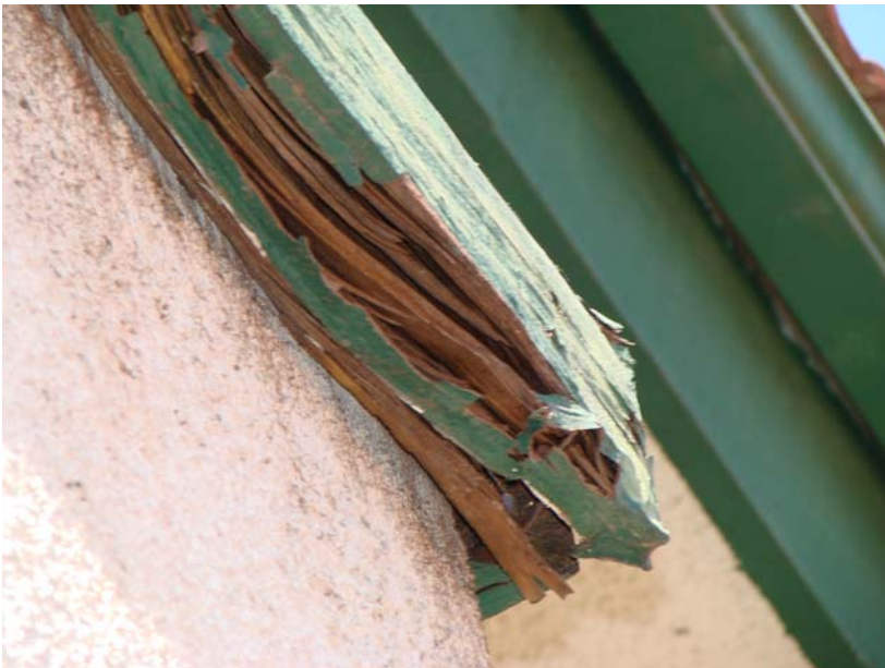
072 P_W: Detail - rotten wood trim on 2nd floor balconies.
