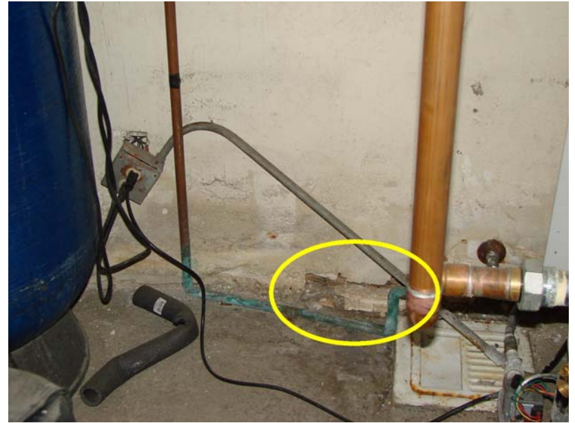
031 P_E: Water damage in water heater closet.
