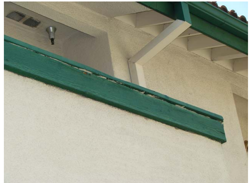
181 P_E: Detail - rotten wood trim on 2nd floor balconies.
