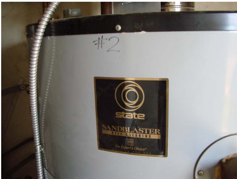
092 P_W: State water heater (#2), 100-gal, 260,000 BTUH.
