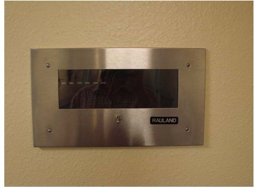
115 P_E: Rauland emergency-nurse call annunciator panel - 2nd floor (South end of West Hall).
