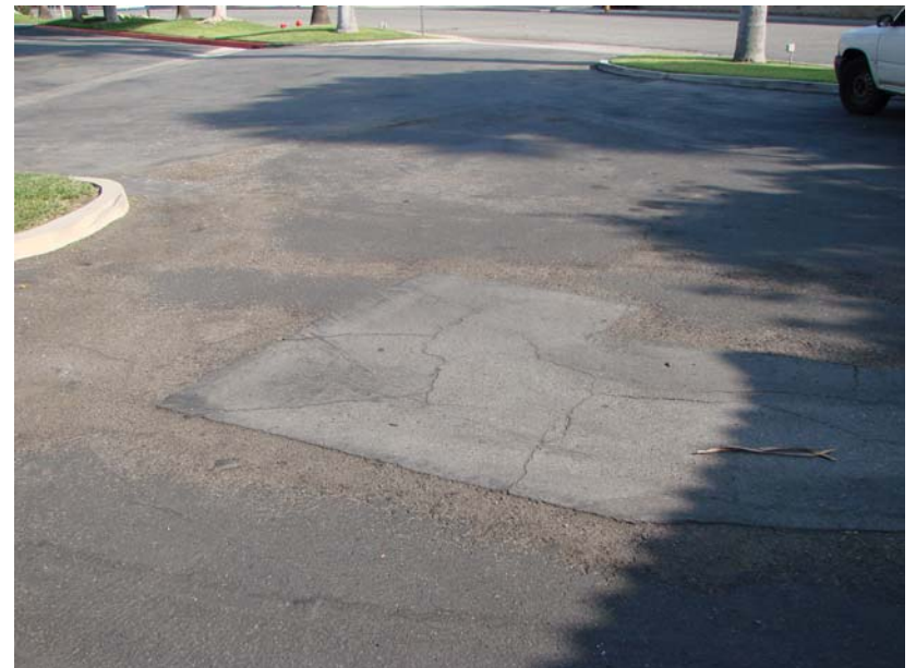
017 P_E: Asphalt paving detail at Palm West - prior asphalt patch.
