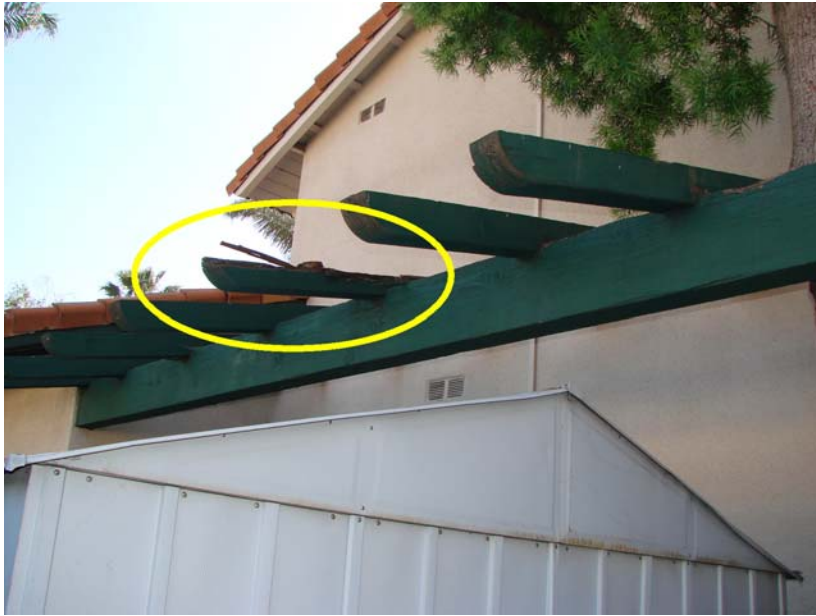
038 P_E: Detail - rotten beam.
