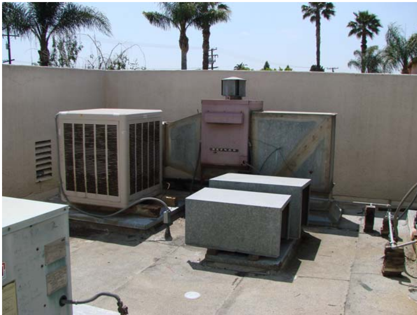
144 P_E: Roof top HVAC units - Kitchen swamp cooler.
