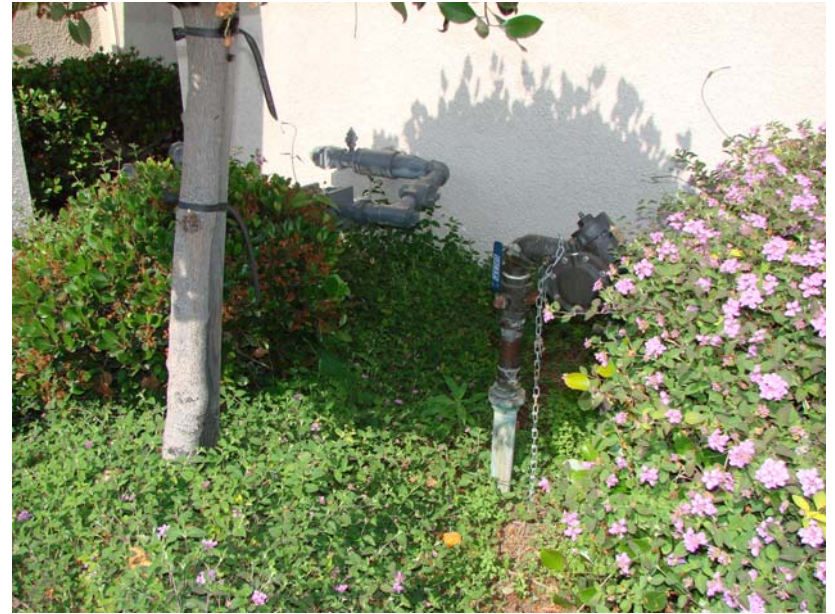
019 P_E: Irrigation sprinkler supply and gas meter.
