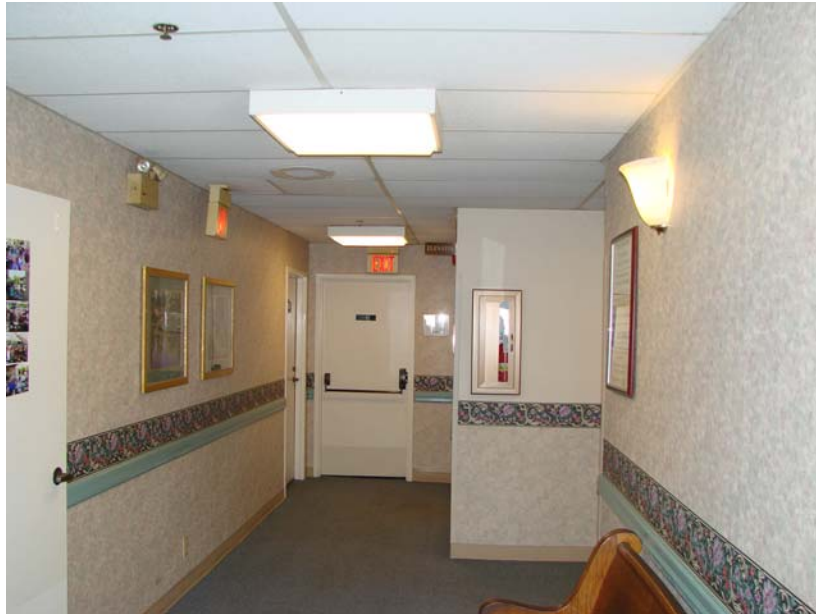
034 P_W: West end of South Hall; elevator. Note batter backup emergency light. Also note carpet, rubber wall base, wall paper, chair rail at handrail height,
