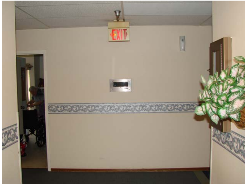
086 P_E: Rauland emergency-nurse call annunciator panel at north end of 1st Floor West Hall.
