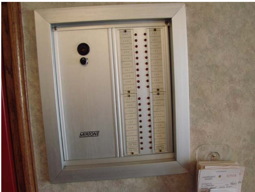
012 P_W: Mirtone emergency call system annunciator panel.
