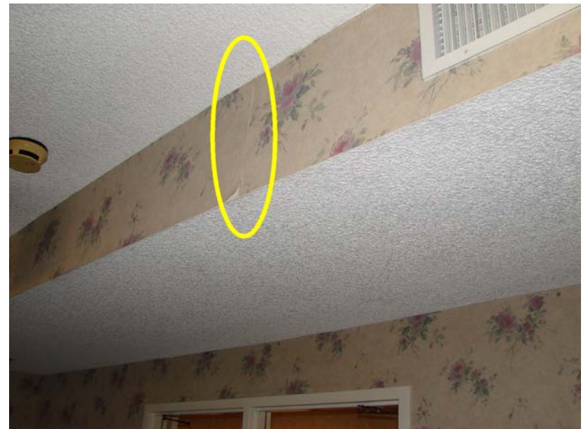
033 P_W: Living room - peeling wallpaper.
