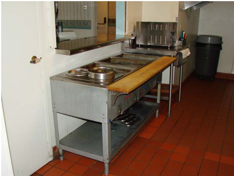
016 P_W: Aerohot steam table - consider replacing.
