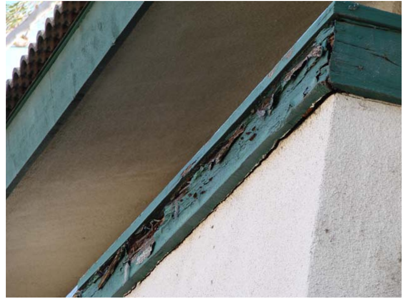
043 P_E: Detail - rotten trim on 2nd floor balcony.
