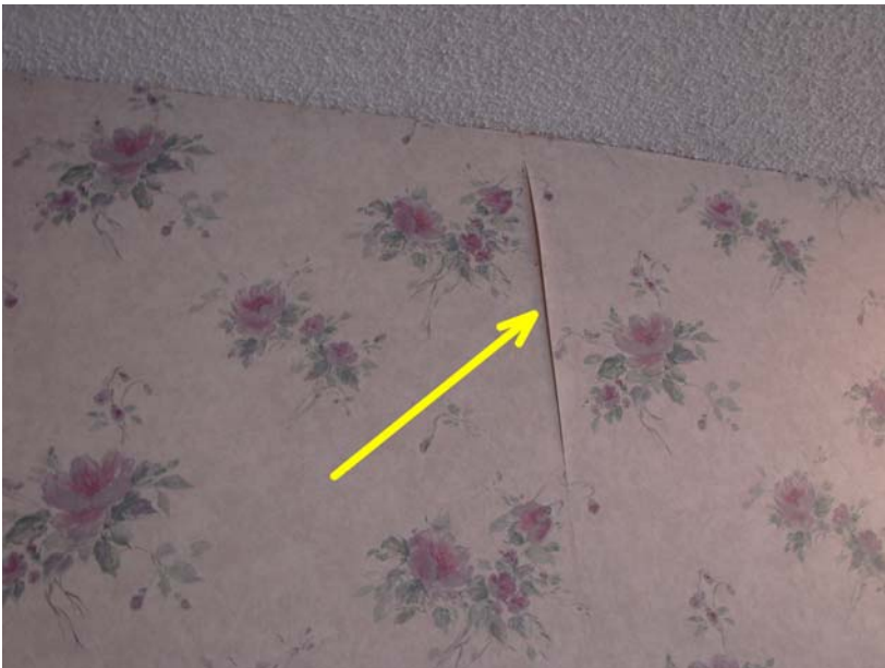
032 P_W: Living room - peeling wallpaper.
