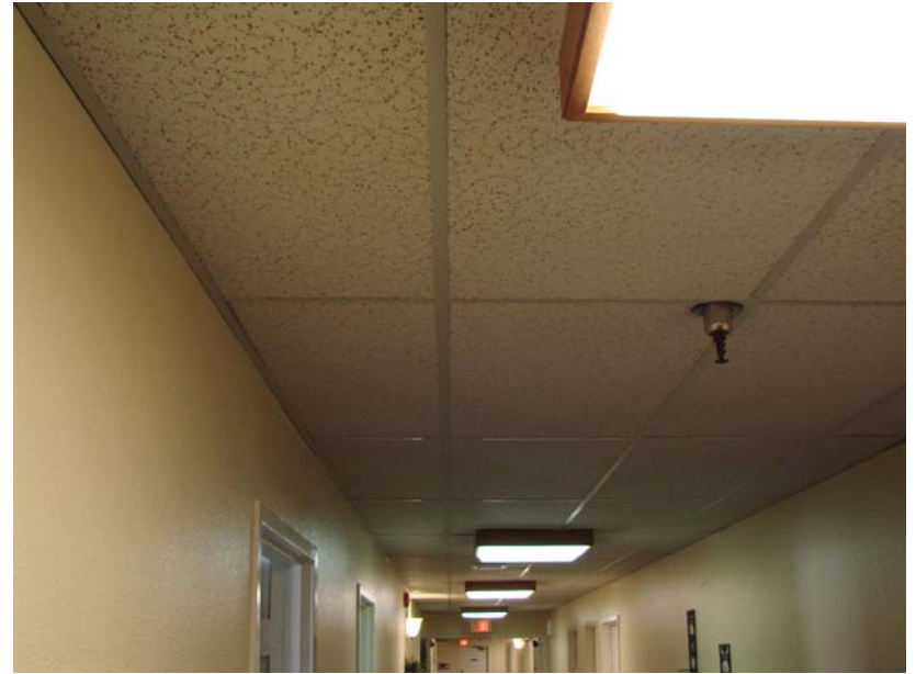
123 P_E: Acoustic lay-in ceiling tile - consider repainting ceiling grid. Replace or paint tile.
