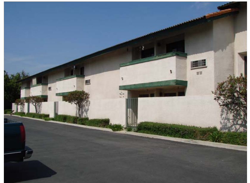
033 P_E: Palm East - west elevation. note rotten wood trim on 2nd floor balconies.
