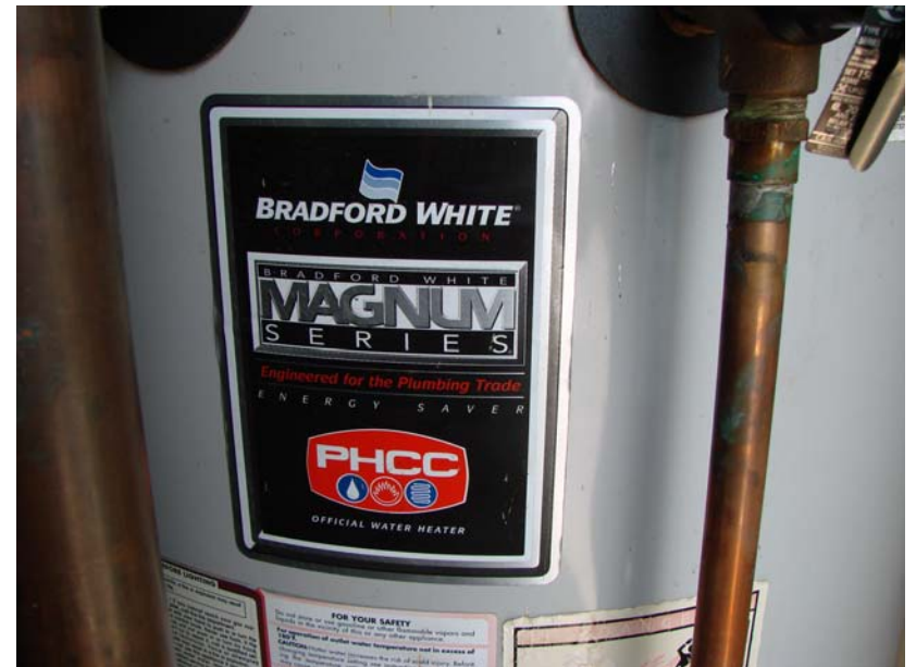
021 P_E: Bradford White water heater (#3), 80-gal, 180,000 BTUH.
