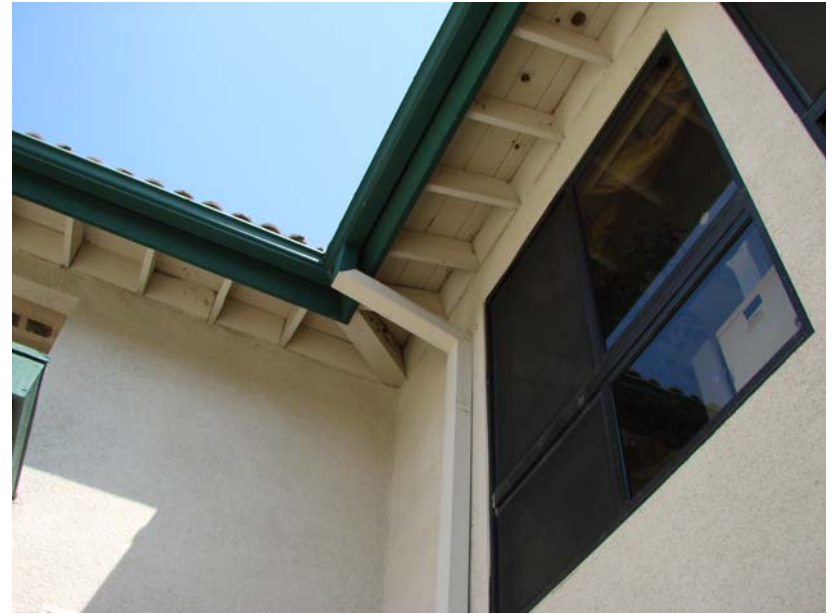
163 P_E: Detail - gutter, wasp nest under soffit.
