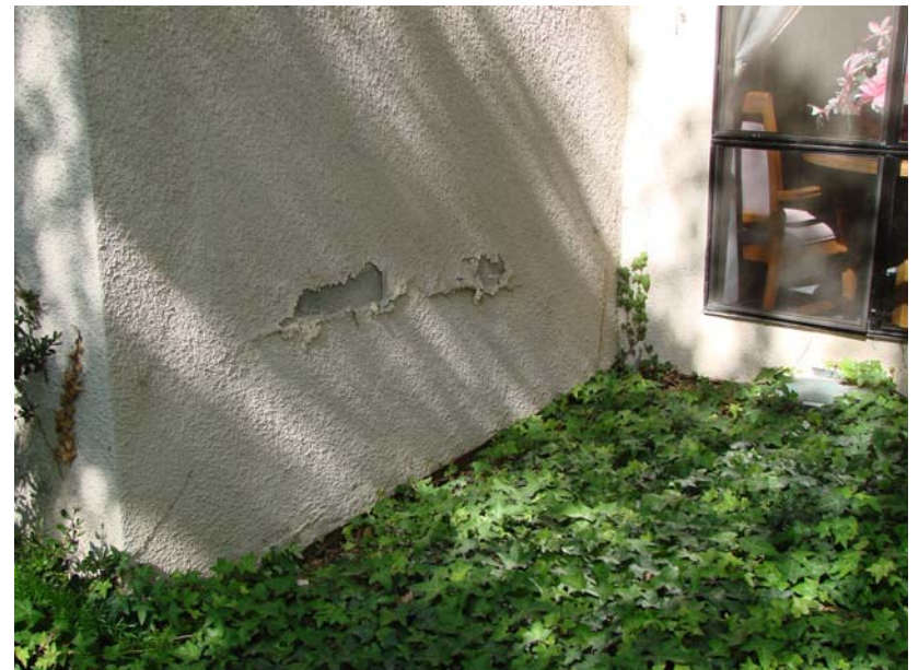
081 P_W: Exterior finish coming off building.
