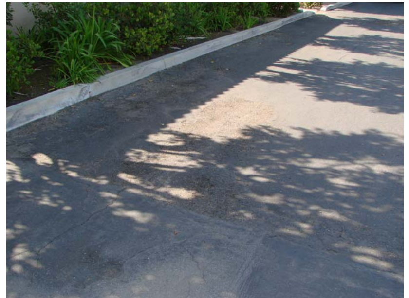
073 P_W: Paving detail - minor surface damage.
