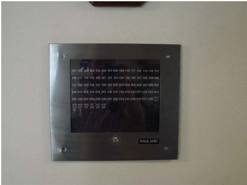
056 P_E: Rauland emergency-nurse call annunciator panel at front entry reception desk.
