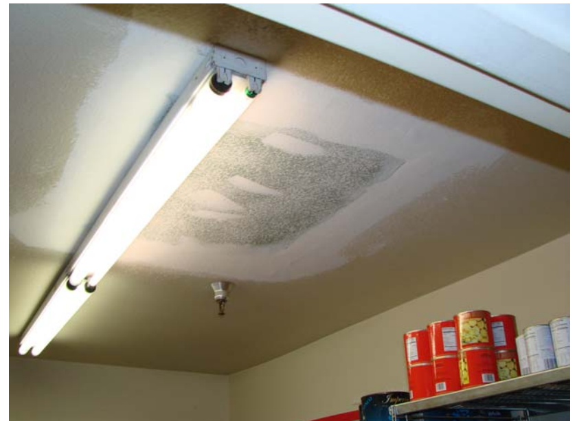
077 P_E: Kitchen - ceiling repair in dry storage (fire sprinkler pipe leak).
