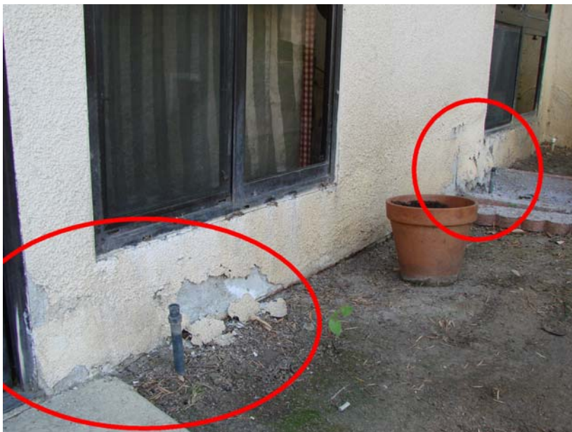
172 P_E: Courtyard detail - water damage outside private dining room (possibly from sprinklers-).
