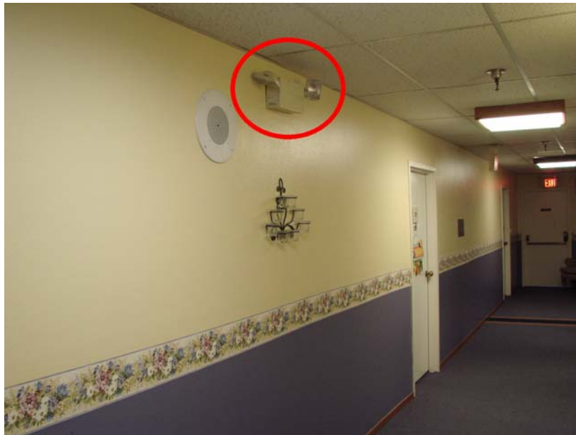
118 P_E: Public Address speaker, battery back-up emergency lighting (no emergency generator).
