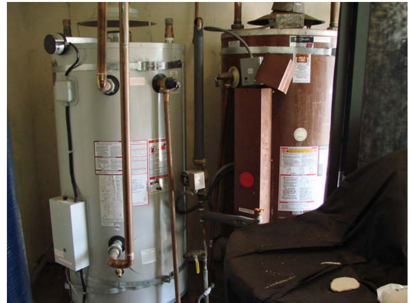
027 P_E: Water heaters #1 & 2.
