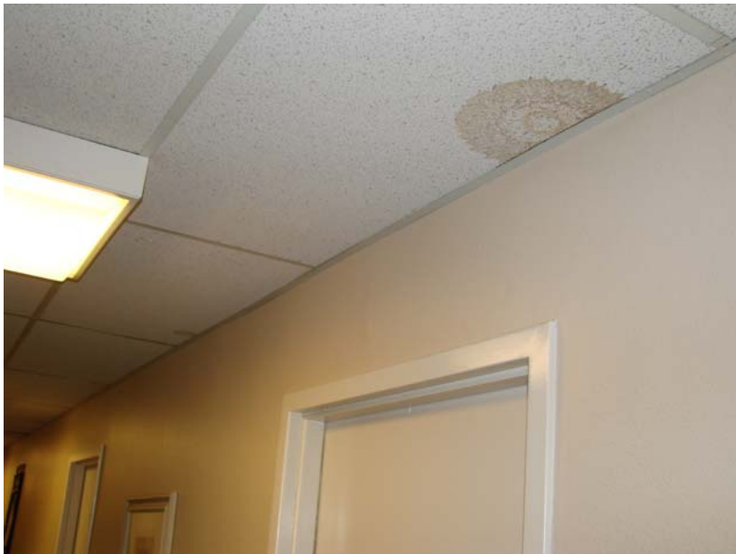
036 P_W: Water stain in 1st floor corridor. Likely from pipe condensation.
