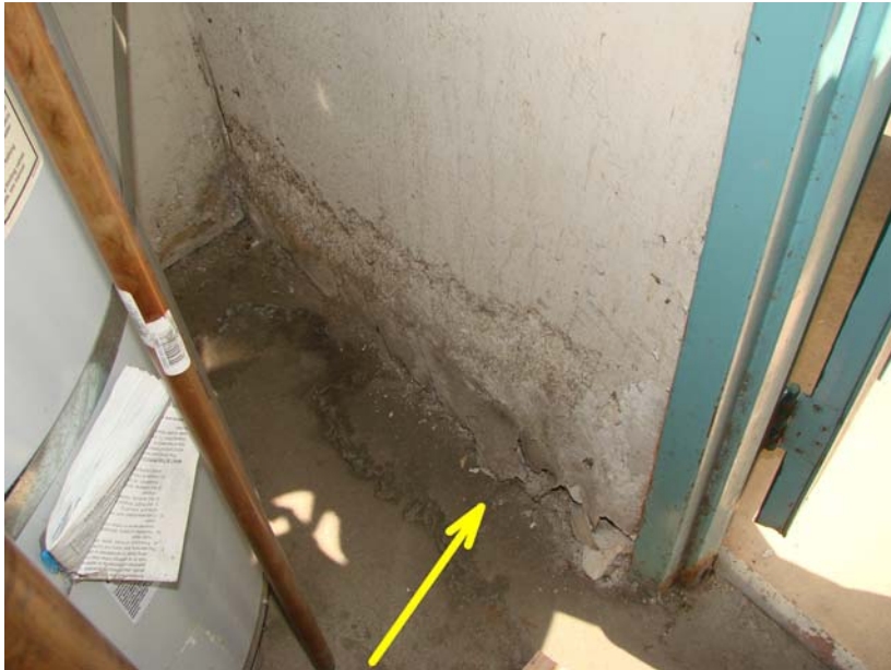
030 P_E: Water damage in water heater closet.
