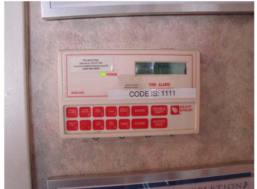
011 P_W: Silent Knight fire alarm annunciator.
