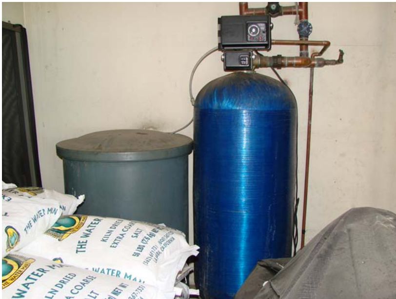
028 P_E: Culligan water treatment system.
