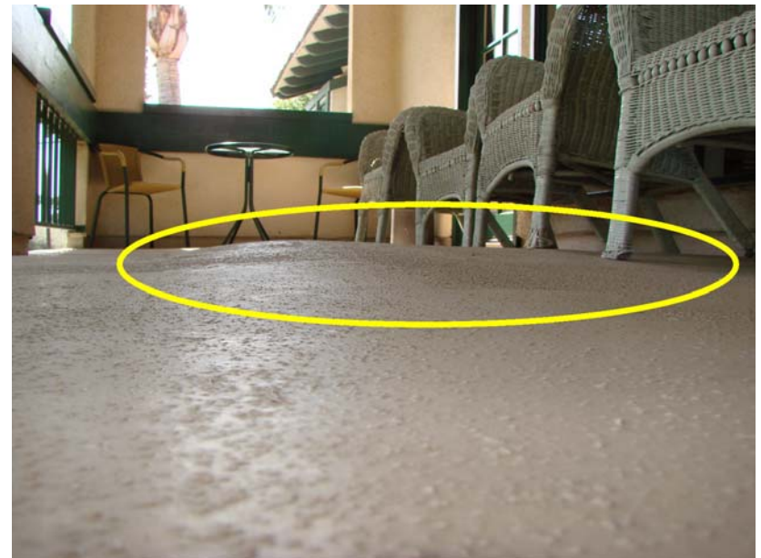
053 P_W: Detail - unusual floor topography on 2nd floor patio.
