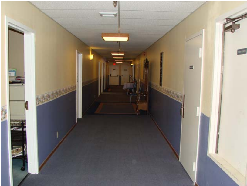
114 P_E: Palm East - typical 2nd floor corridor. Wood base, painted walls, no handrails, wallpaper border transition. Paint and border are currently being
