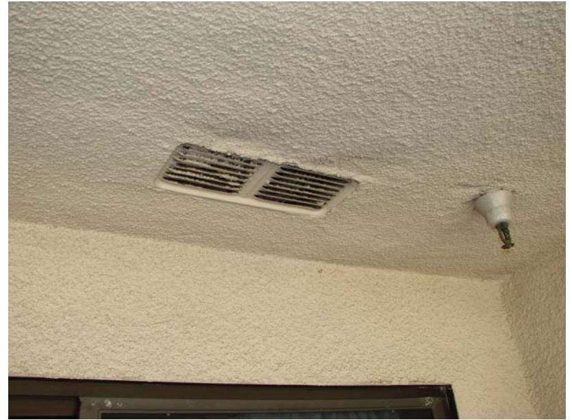
175 P_E: Soffit vent - needs to be cleaned.
