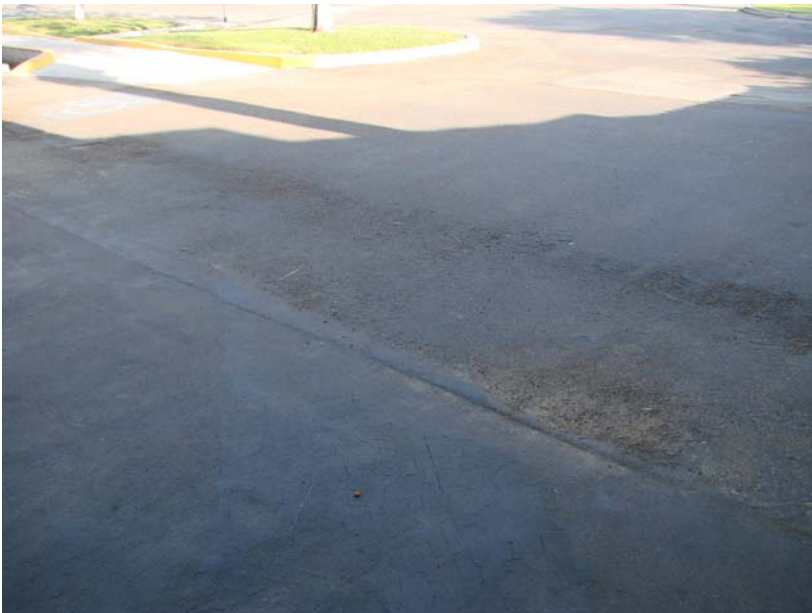
016 P_E: Asphalt paving detail - minor surface damage.
